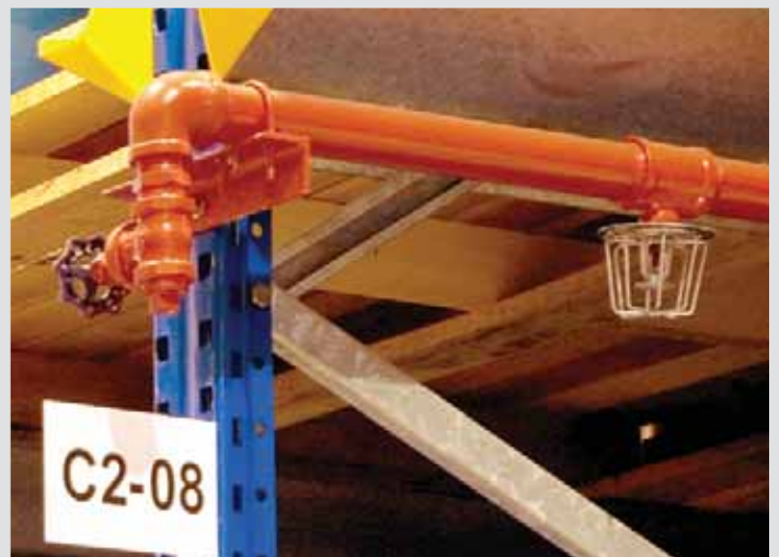
Sprinkler heads may be located within the racking, or in the gap between 2 sides of double faced rackings
